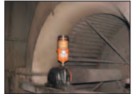
Grease lubricator installed on a blower fan
