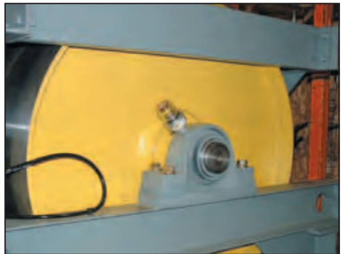
Grease lubricator installed on pillow block of a dynamometer
