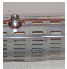
Earthing can thus be fitted every 4 metres to save 25% of time and earth connector installation.
