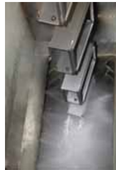
Pressurized Spray Cleaning Line
