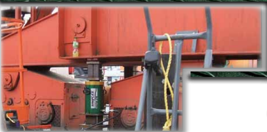
Simplex 150 ton aluminum locknut spring return cylinders are used to lift this large crane for routine maintenance on bearings.
