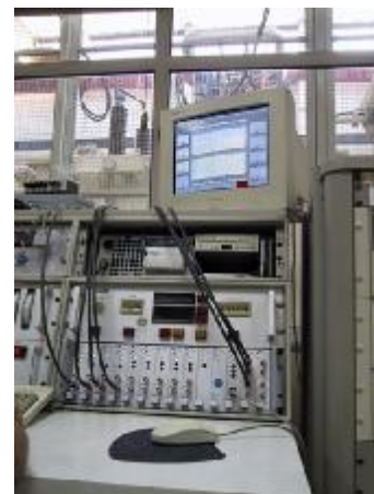
ICMsys8 installed in a control room
