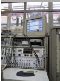
HV control room
