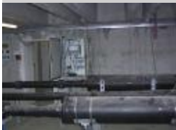
400 kV cable joints
