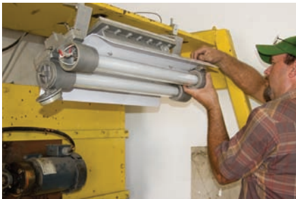
4. Replace with a new globe assembly in the reverse order. Feed the wires back into the globe ends & bolt in place.
