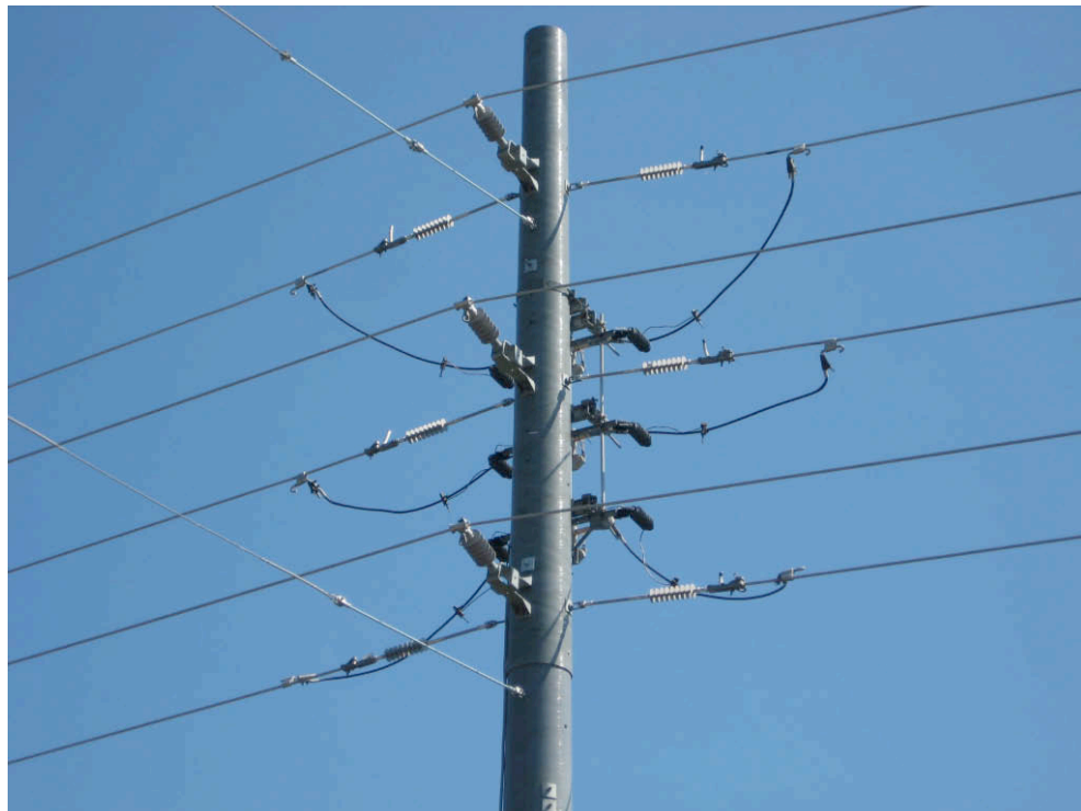
Extension Insulator Application with Load Interrupter Switch Installed
