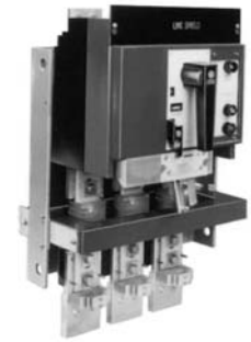
HPC Switches with Integral Ground Fault Protection
