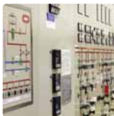
Medium voltage energy distribution
