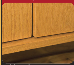
Cabinet doors won't stay even with the surface
