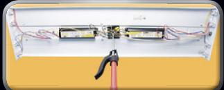
Hanging light fixtures
