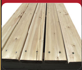
Misaligned screws & unevenly spaced splintered boards
