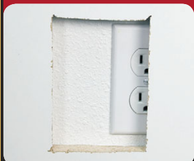
Cut in the wrong place
