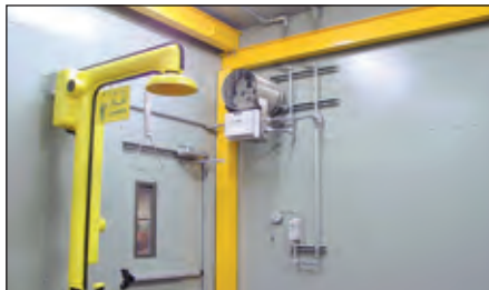
Emergency shower for personnel safety
